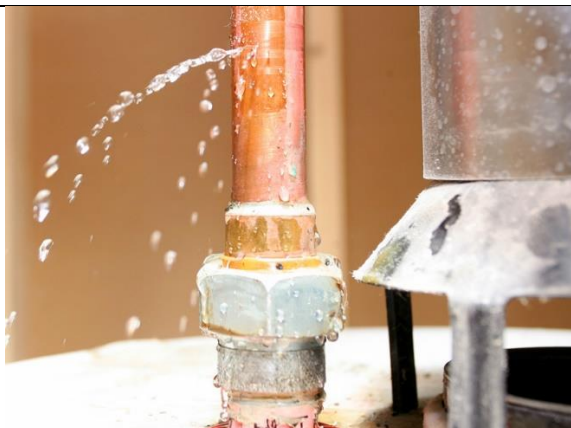
Slika: Počena cev (24-Hour Emergency Plumbing Service, 2020).
